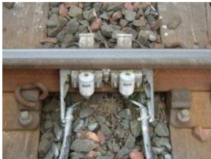
Figure (2.5) an axle counters detection point, in the UK
