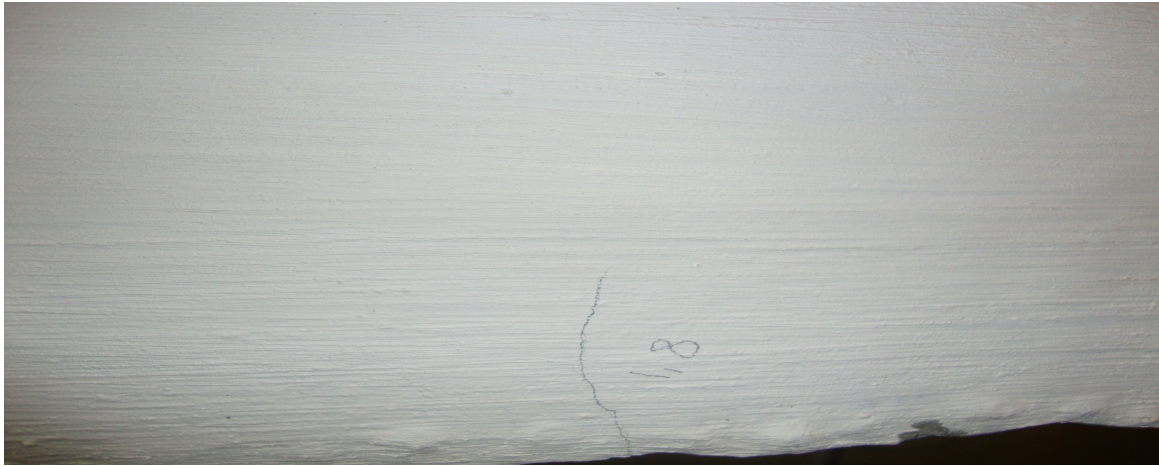
C8 - First Cracking
