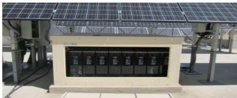
Figure 3.6: Battery box's overview
