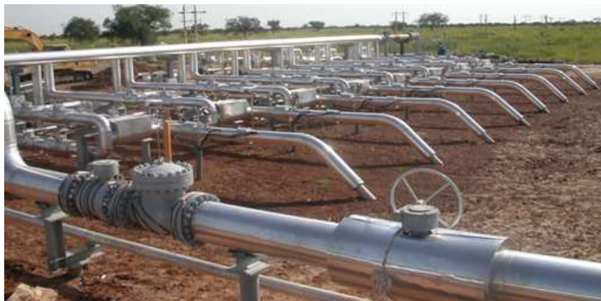
Figure C.2: Production Header - Oil Gathering Manifold.
