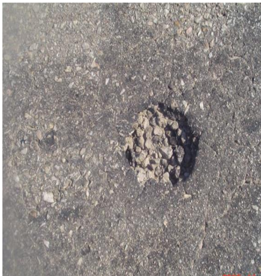
Figure 3.32 Low Severity Potholes
