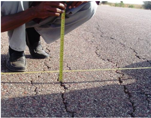
Fig. 3.16: Low Severity Depression
