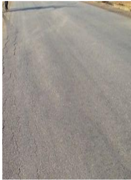
Fig. 3.11: Medium Severity Upheavals and Settlements
