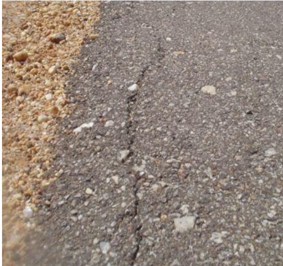
Fig. 3.19: Low Severity Edge Cracking
