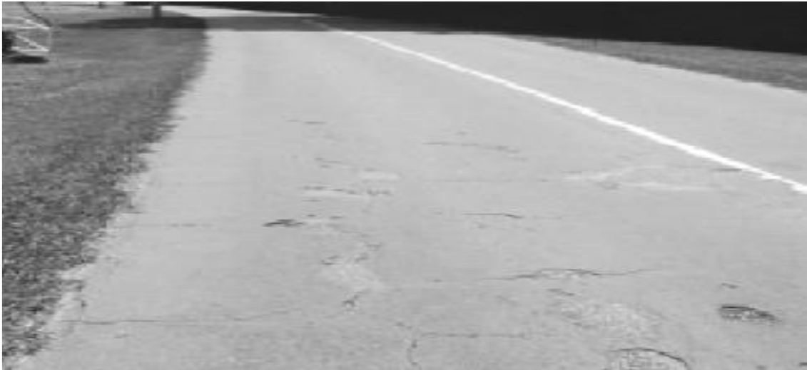
Figure 3.37 High Severity Raveling
