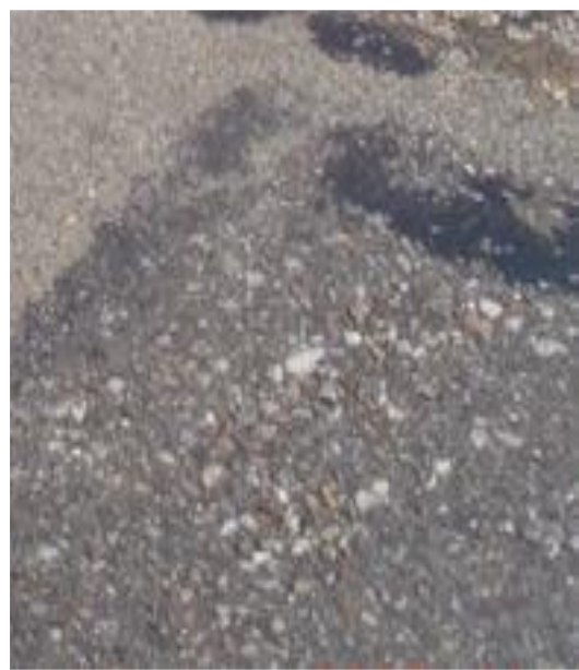
Fig.3.29: Medium Severity Patching
