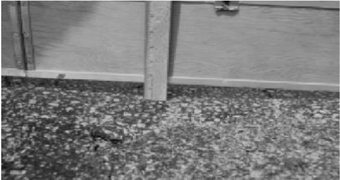
Figure 3.43 High Severity Rutting
