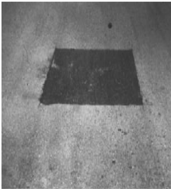
Fig. 3.28: Low Severity Patching
