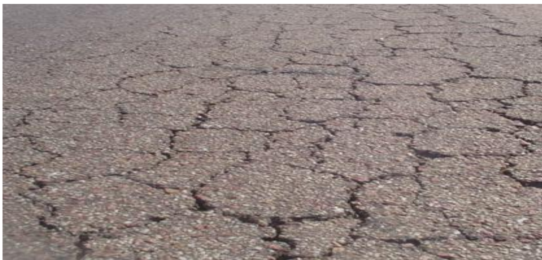
Fig. 3.3: High Severity Alligator Cracking
