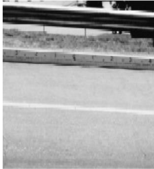
Fig. 3.14: Medium Severity Corrugation
