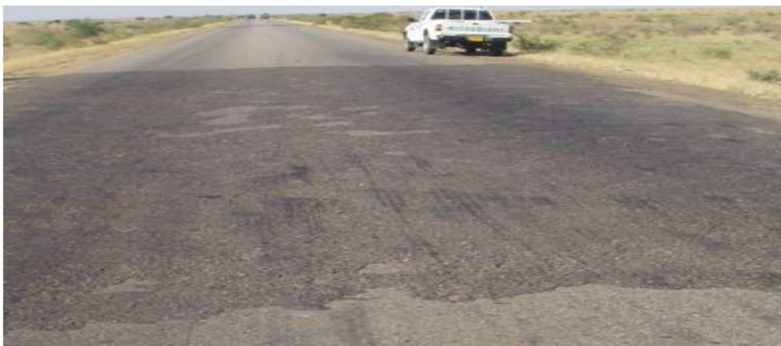
Fig. 3.30: High Severity Patching
