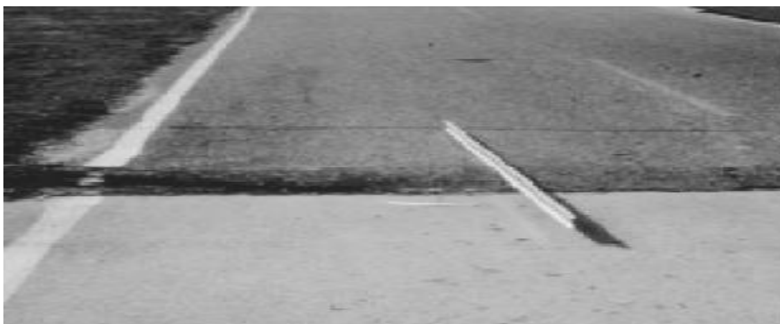
Figure 3.46 high Severity shoving
