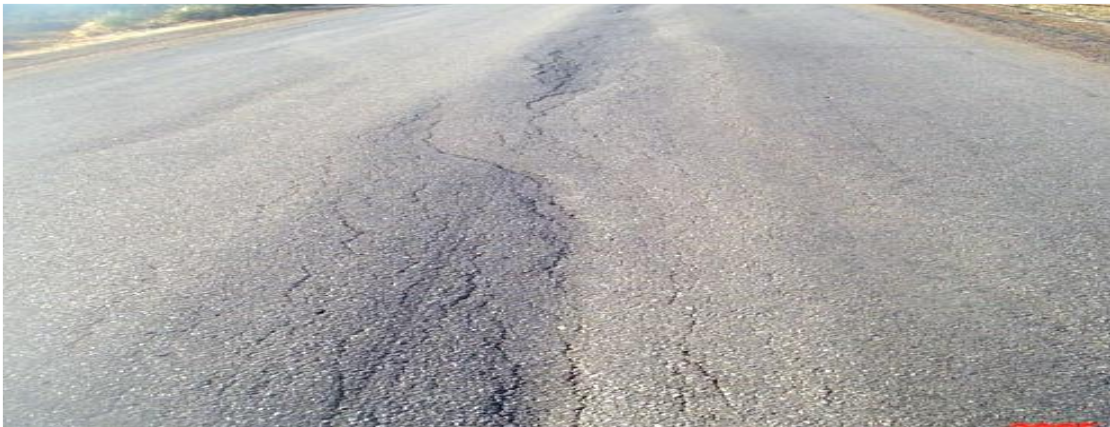
Fig. 3.12: High Severity Upheavals and Settlements
