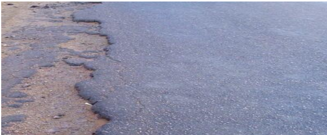
Fig. 3.21: High Severity Edge Cracking
