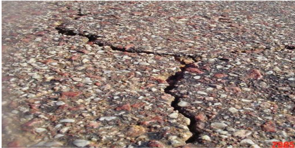
Fig.3.9: High Severity Block Cracking
