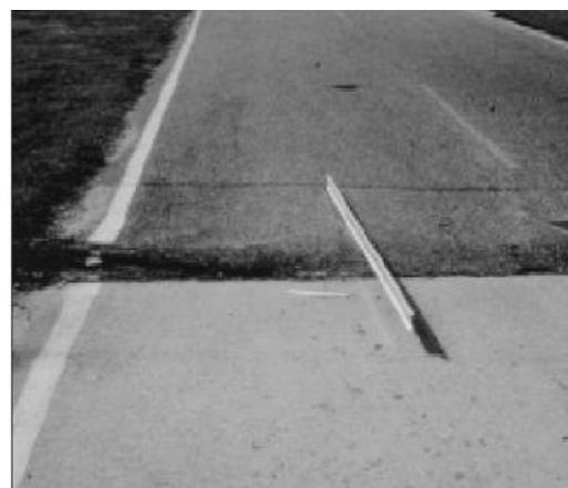
Figure 3.45 Medium Severity shoving
