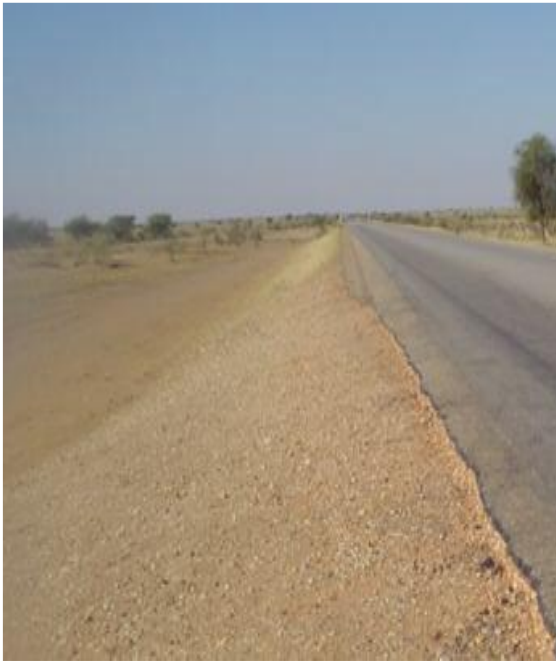
Fig. 3.22: Low Severity Lane/Shoulder drop-off
