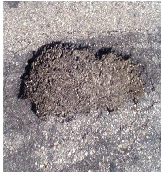
Figure 3.33 Medium Severity Potholes
