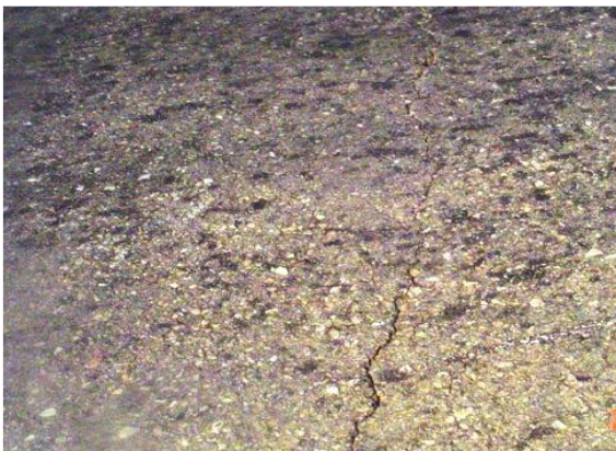
Figure 3.38 low Severity reflection cracks
