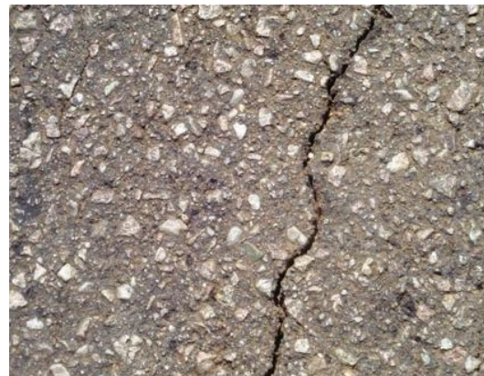
Figure 3.39 medium Severity reflection cracks
