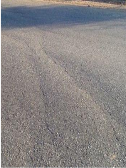
Fig. 3.10: Low Severity Upheavals and Settlements
