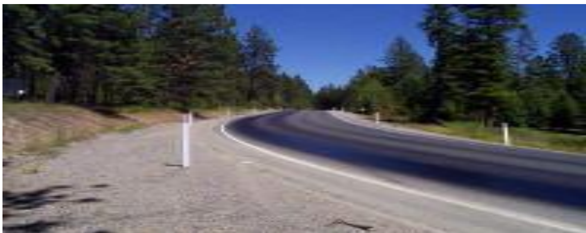
Fig. 3.6: High Severity Bleeding
