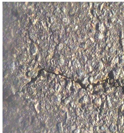
Fig. 3.26: Medium Severity Longitudinal and Transverse Cracking
