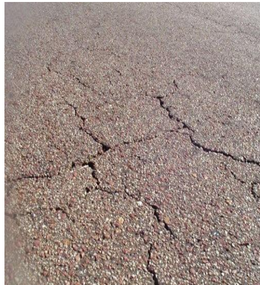
Fig. 3.8: Medium Severity Block Cracking
