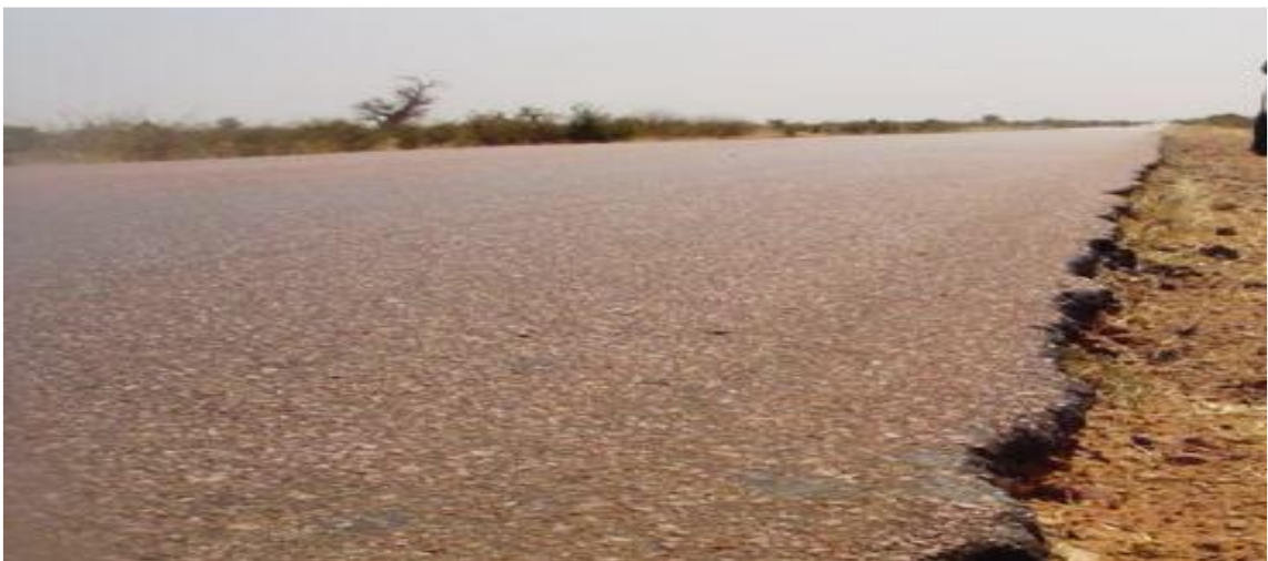
Fig. 3.24: High Severity Lane/Shoulder Drop-off
