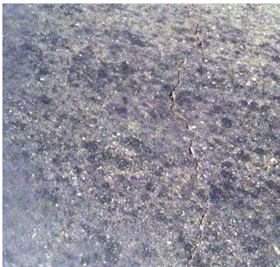
Fig. 3.25: Low Severity Longitudinal and Transverse Cracking
