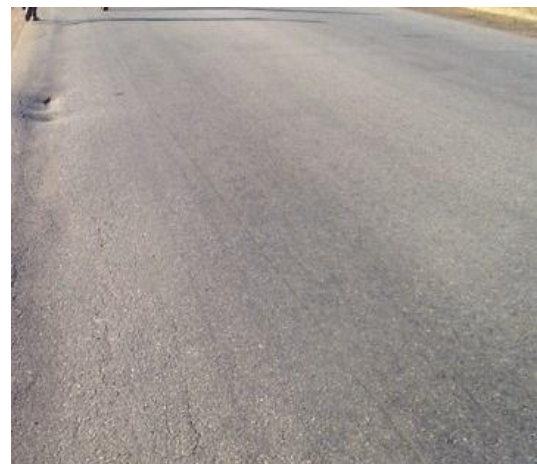
Figure 3.42 Medium Severity Rutting
