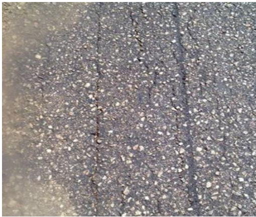
Fig. 3.1: Low Severity Alligator Cracking
