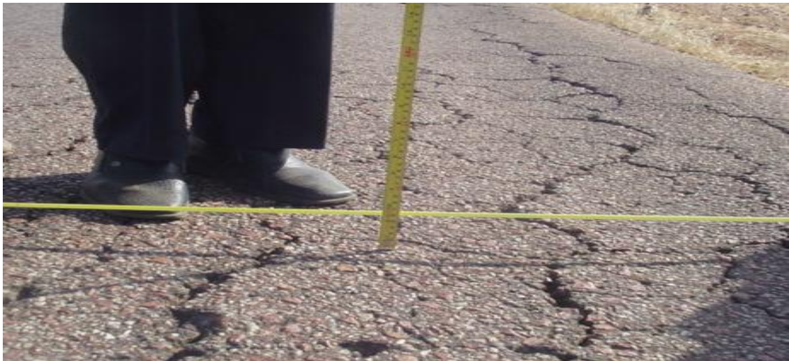
Fig. 3.18: High Severity Depression
