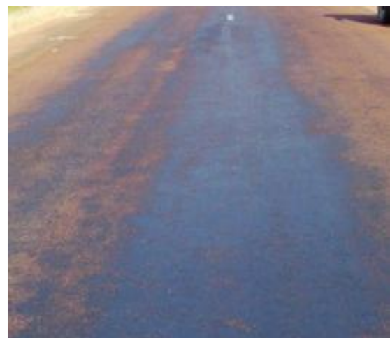
Fig. 3.5: Medium Severity Bleeding
