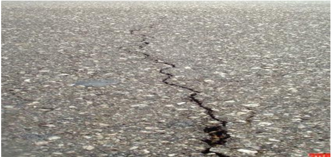
Figure 3.40 High Severity reflection cracks
