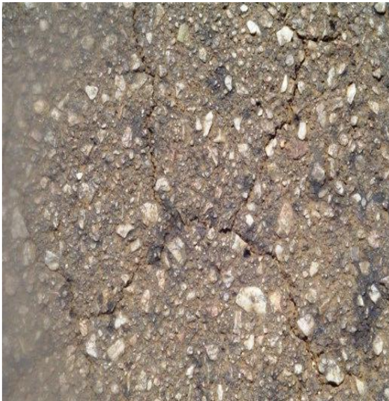
Fig. 3.7: Low Severity Block Cracking
