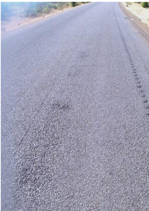
Figure 3.35 Low Severity Raveling
