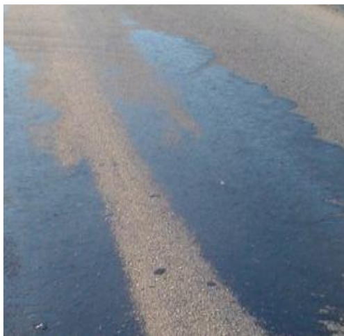
Fig. 3.4: Low Severity Bleeding
