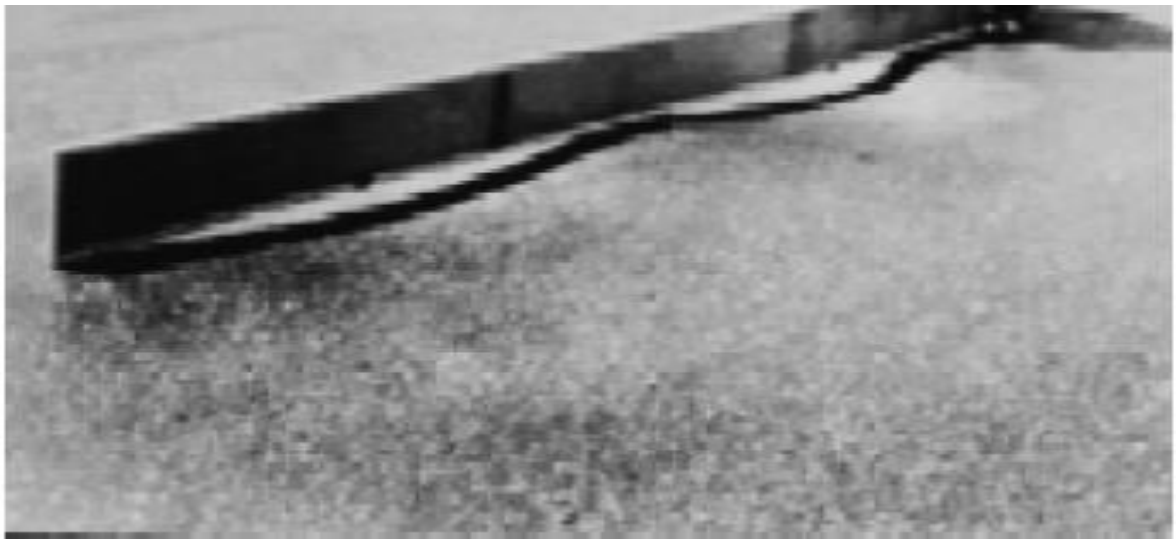
Fig. 3.15: High Severity Corrugation
