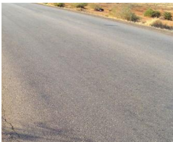
Figure 3.41 low Severity Rutting
