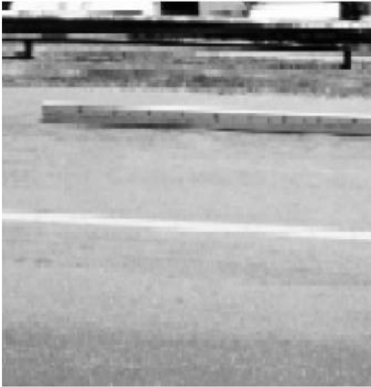
Fig. 3.13: Low Severity Corrugation
