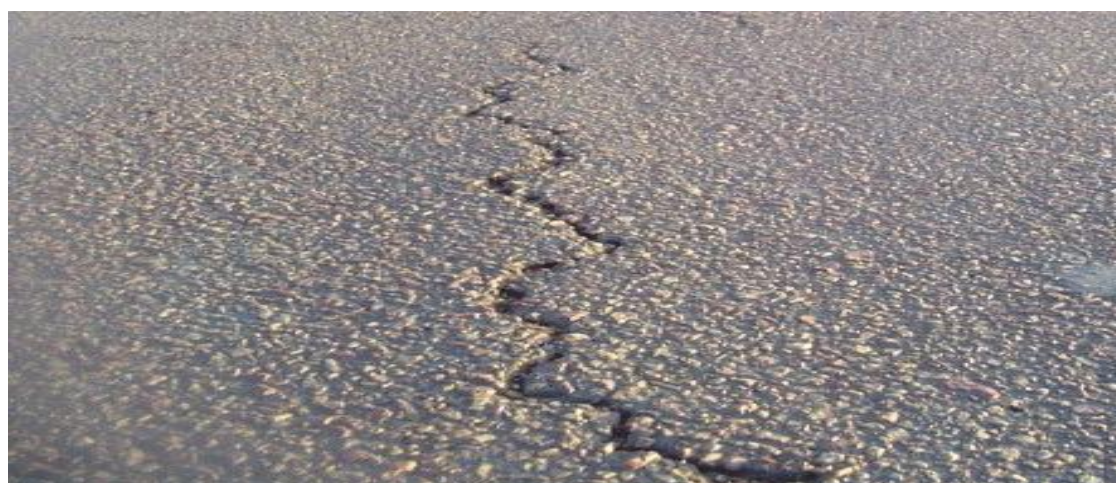
Fig. 3.27: High Severity Longitudinal and Transverse Cracking
