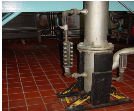
Figure 4.2 simple example of a sight glass
