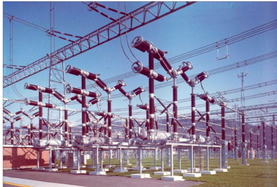
Fig(3.1) AIS Substation
