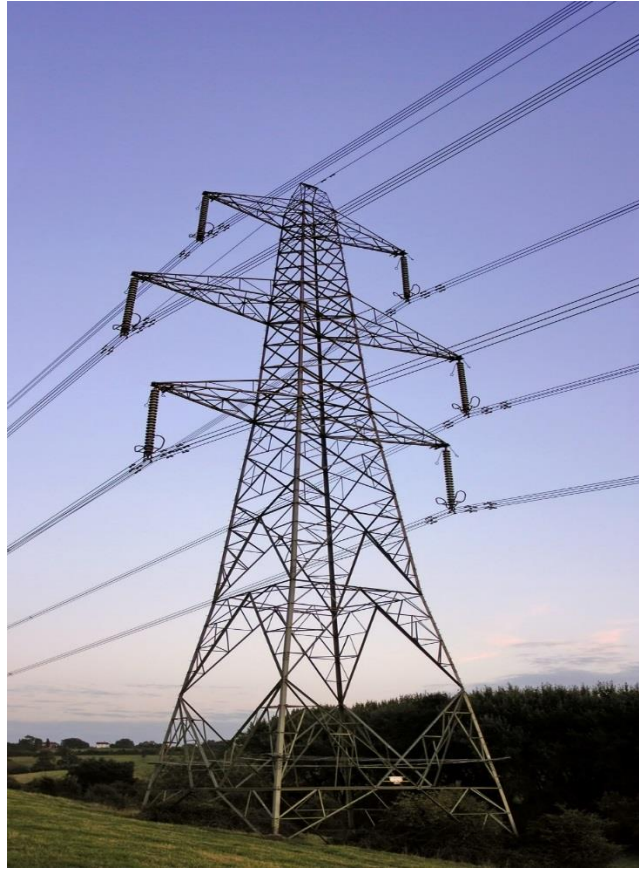
Figure 2.7: Suspension steel tower.
