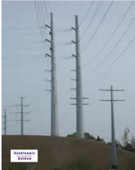
Figure 2.11: Tubular steel poles.
