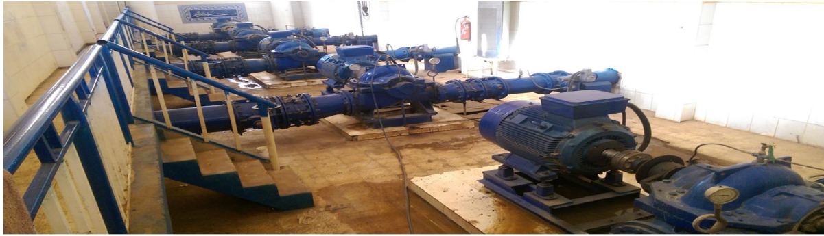
Figure 3.1 for ALSAHAFA pumping Station (KSWC)
