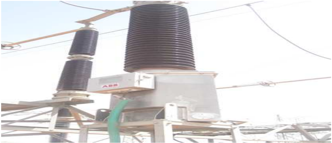
Figure 3.3: Voltage transformer and Current transformer
