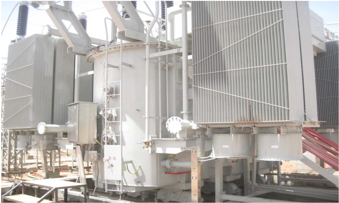
Figure 3.9: The Main Transformer 220/110/11KV
