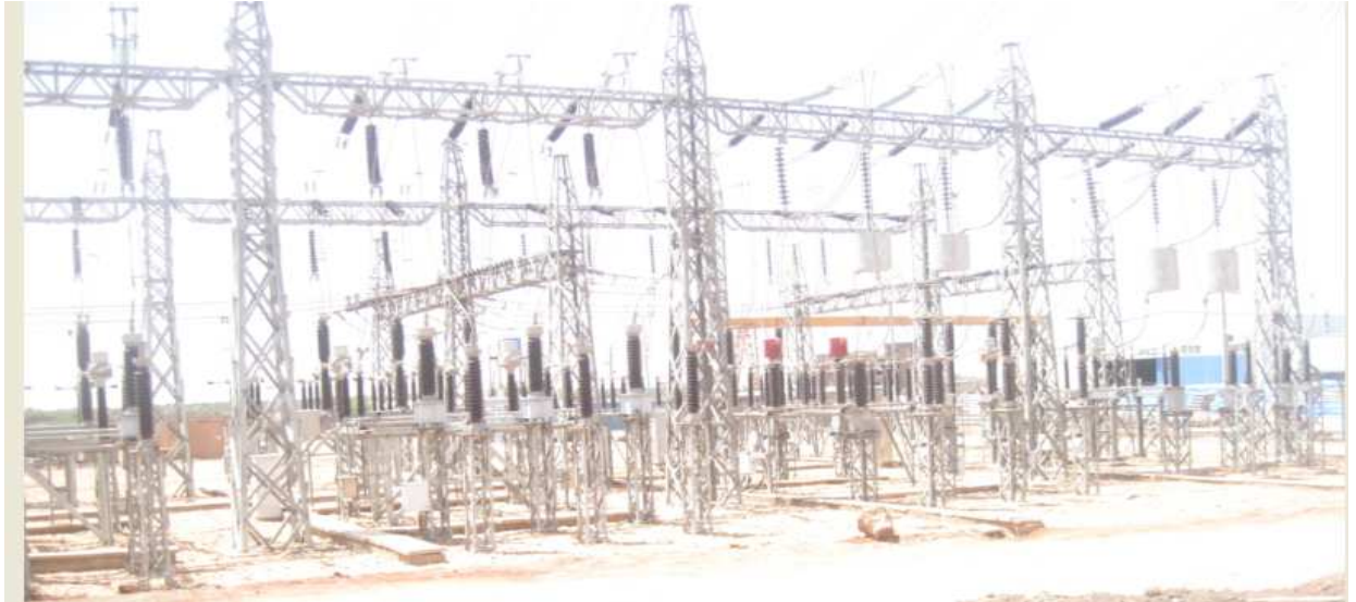
Figure 3.1: General view of Kilo-X Substation
