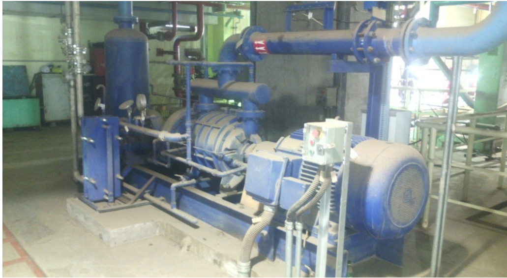
Fig (3.3) show the vacuum pump for BAHRI STATION PHASE III
