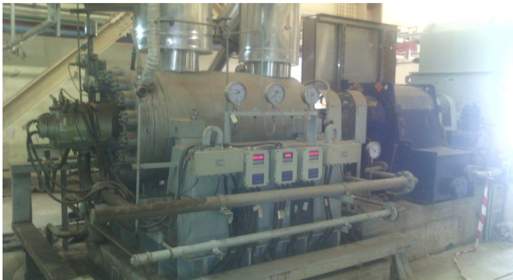
Fig(3.5) Boiler Feed Pump BAHRI STATION PHASE III
