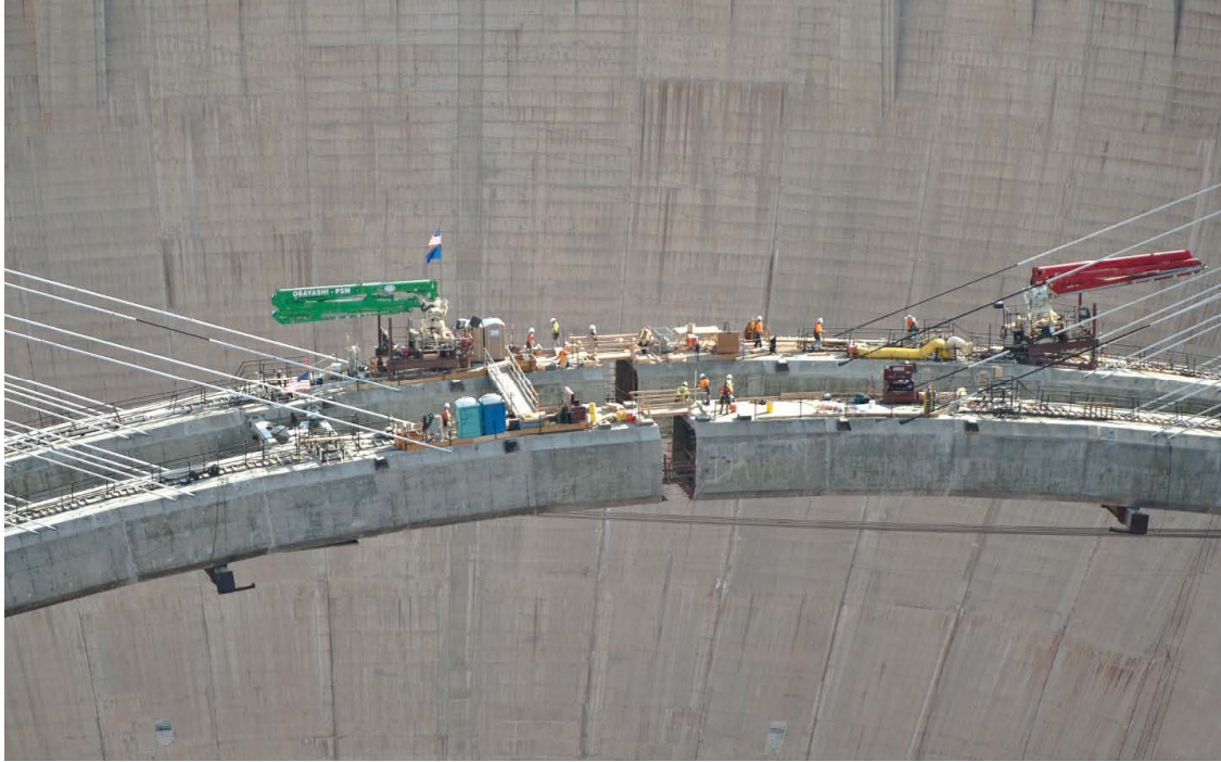
Figure 2.3: ROAD& BRIDGE CONSTRUCTION hazard (9)
