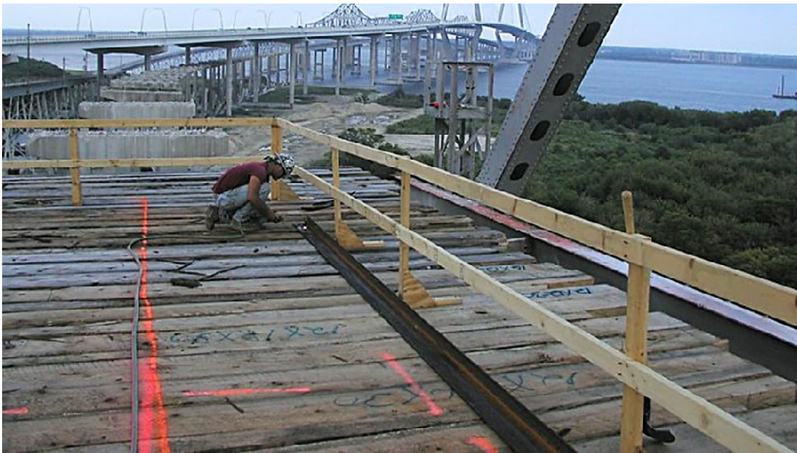
Figure2.2.3 two construction worker fall to their death through temporary wooden bridge platform Photo credit: C. Frank Starmer and Sparky Witte from http://oldcooperriverbridge.org
