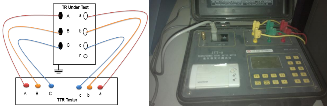
Figure 3.7 shows test set and connection circuit for turn ratio test
