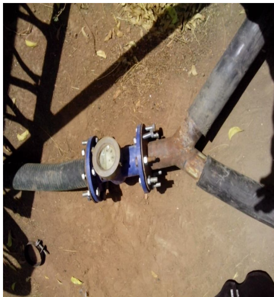
(plate3.7): Flow meter connected to pump and tank (3inch)
