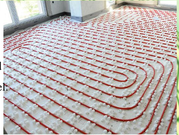
Figure 5-22: hydronic system view
