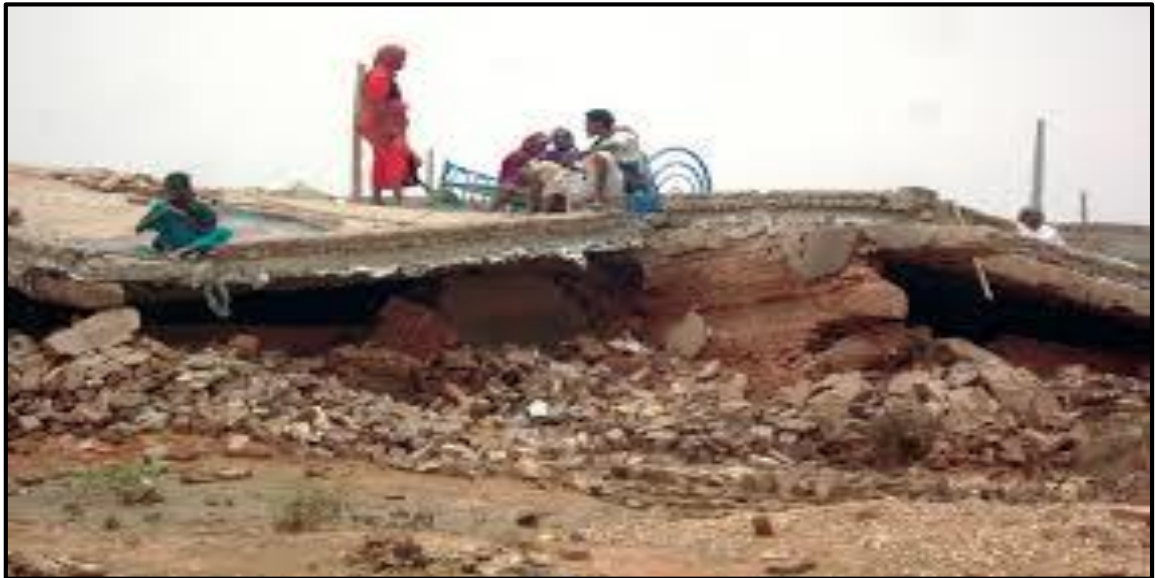
Figure (1-3): Collapse of buildings made of strong building materials
