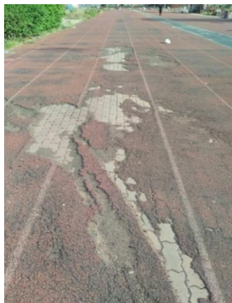
running track has a lot of cracks
