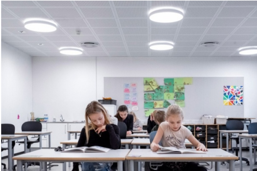
Fig 2.14- electrical lighting in a classroom
