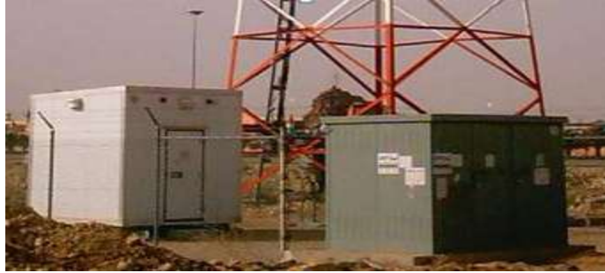
Figure (2.22) a picture of types of base stations attached to towers.
