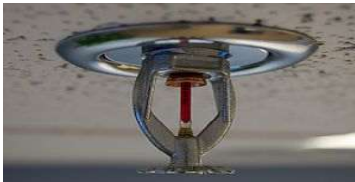
Figure 2-6: Fire Sprinklers System
