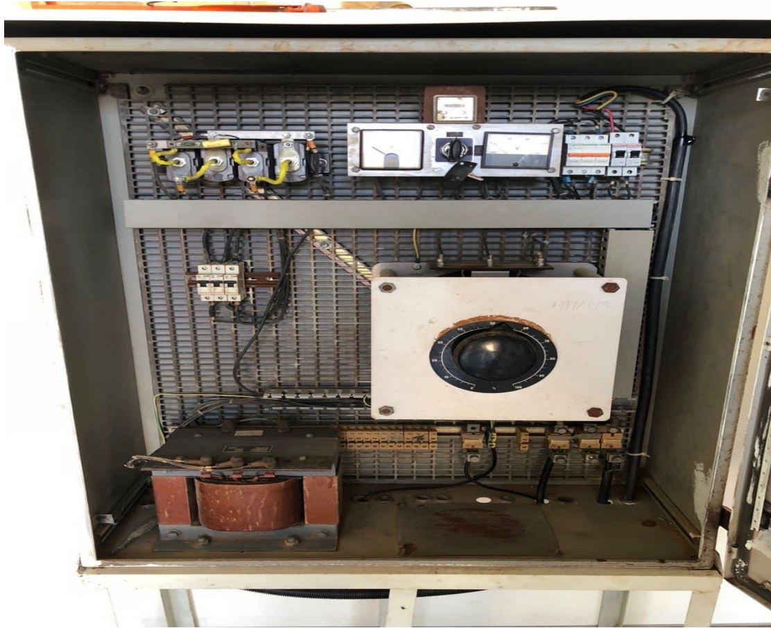
Image shows rectifier for AC power
