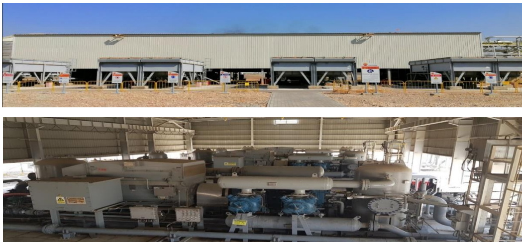
Figure [3.6] The compression units and Ariel coolers
