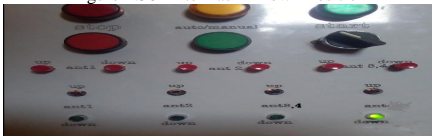
Figure 4.37 Indicating Antennas in Down Position
