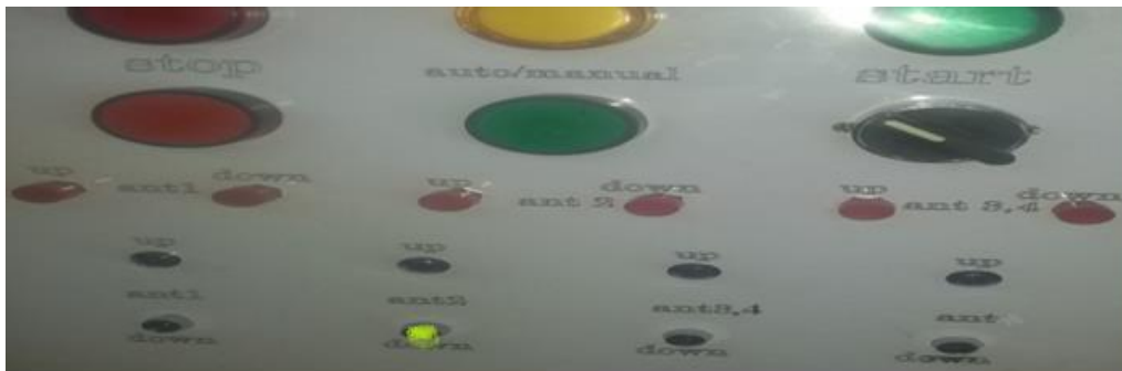
Figure 4.53 Indicator of Antenna 2 Moves to Dawn Position
