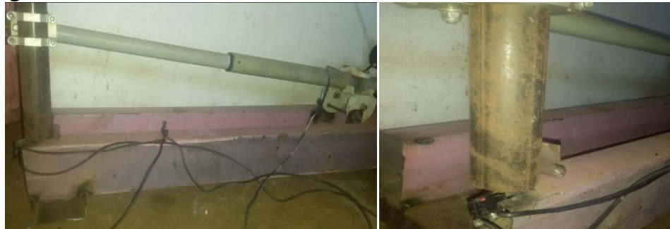
Figure 4.40 Antenna1 Moves to Up Position
