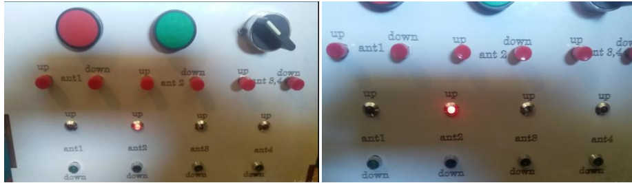
Figure 4.45 Antenna2 Moves to Up Position
