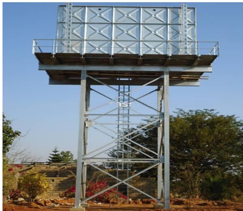
Figure 2.5 Water storage tank
