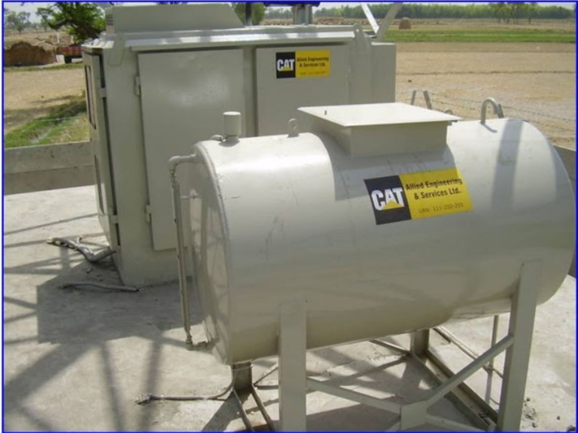
Figure 3.8: Back up generator with fuel tank
