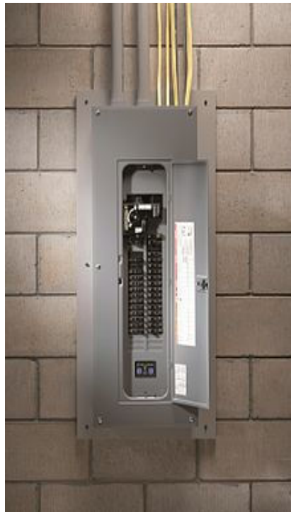
Figure 2.6: Intelligent Transfer Switch
