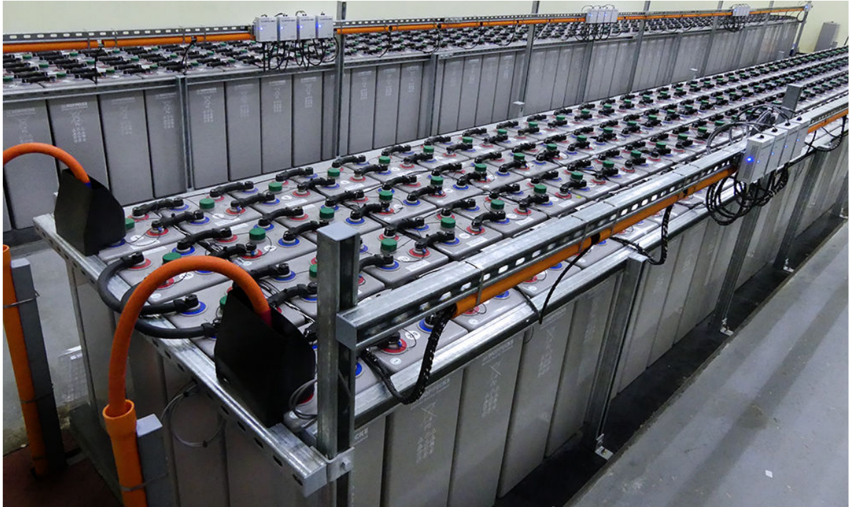
Figure 2.5: battery management for large scale energy storage
