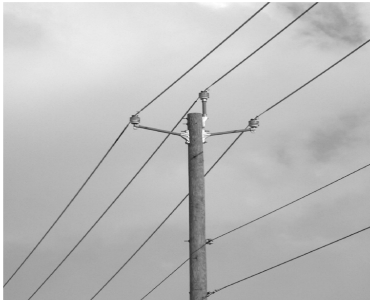
Figure (2.7): overhead distribution structures
