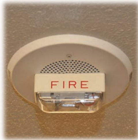
Figure 3.2 a ceiling-mounted re alarm speaker and strobe light Combination unit.
