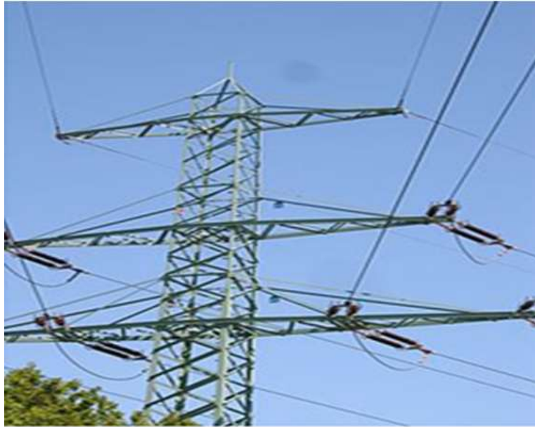
Fig (2.1) Transmission Line 110KVA
