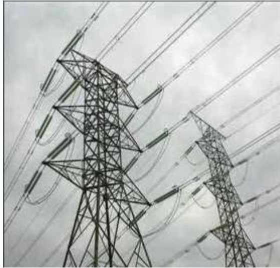
Fig (2.4) Tension Towers
