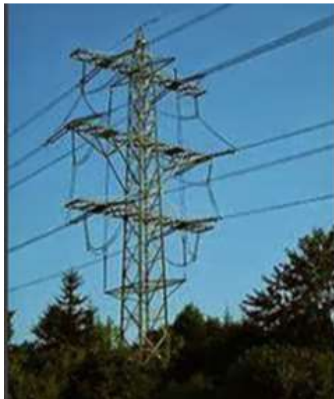
Fig (2.8) Transposition Towers
