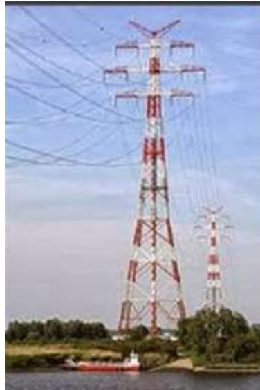
Fig (2.6) Crossing Towers
