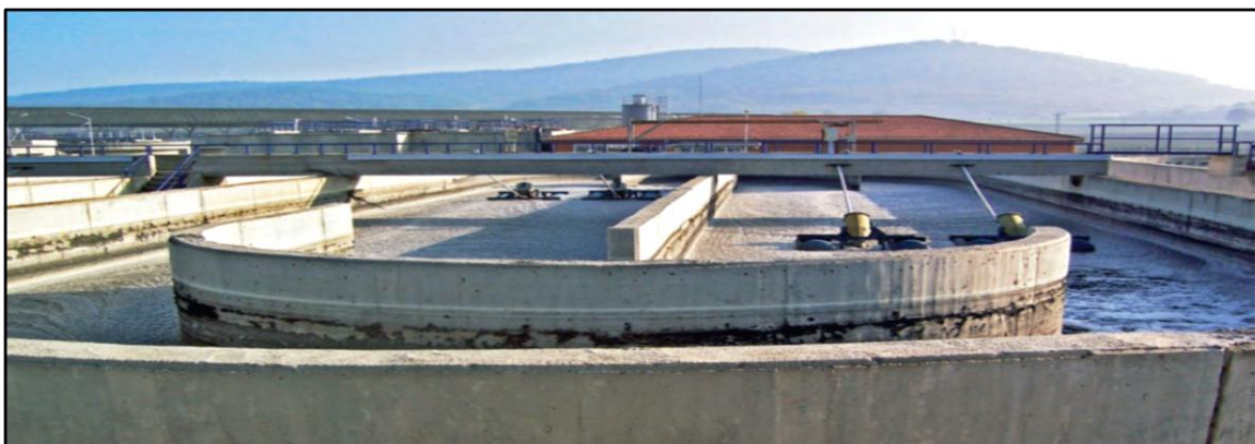
Figure (2-24): Oxidation ditch in operation Oxidation ditch in operation [A. Itodo1, 2018].
