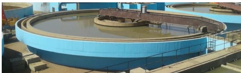
Fig (4.13): Sedimentation basin at Mogran Water Plant.
