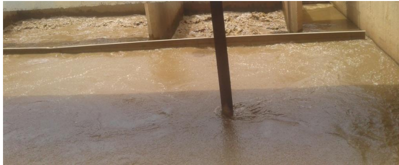
Fig (4.17): Flash mixing basin at Bahri Water Treatment Plant.
