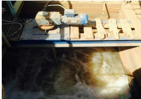
Fig (4.12): Flash mixing at Mogran Water Plant.
