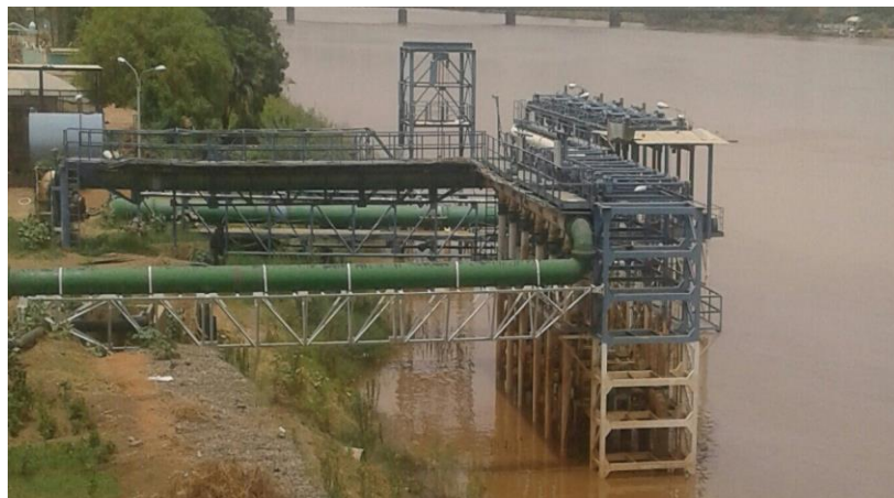
Fig (4.16): Intake at Bahri Water Treatment Plant.
