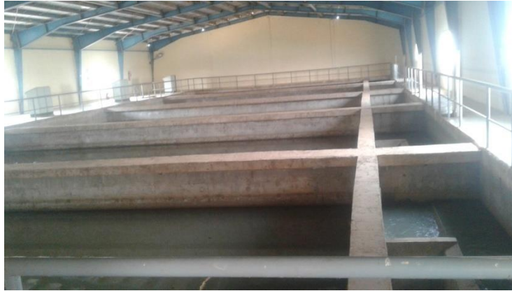
Fig (4.7): Rapid sand filters at Jabal Awlia Water Treatment Plant.
