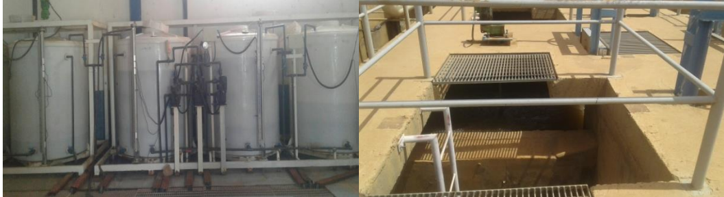
Fig (4.5): Pac dosing chambers and flash mixing at Jabal Awlia Water Treatment Plant.
