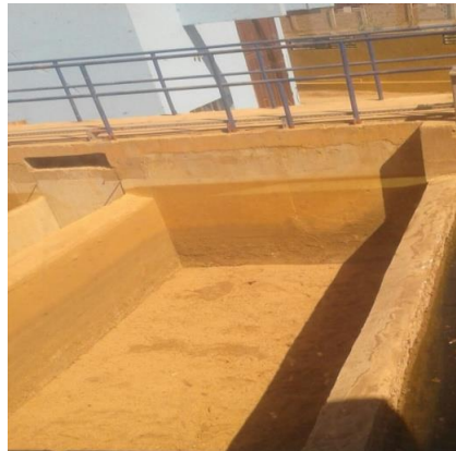
Fig (4.14): Rapid Sand Filter at Mogran Water Treatment Plant.
