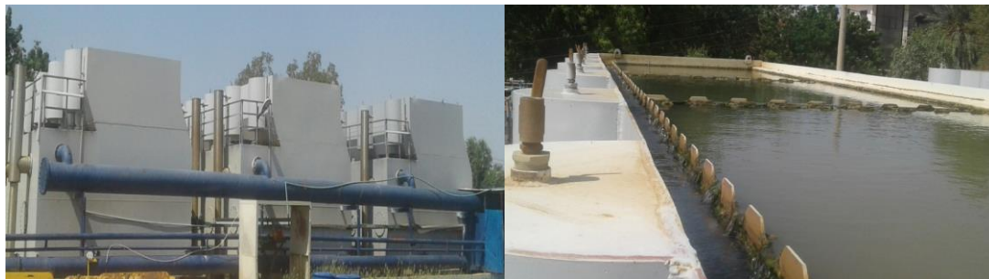
Fig (4.2): Treatment units at Alshajra Water Treatment Plant
