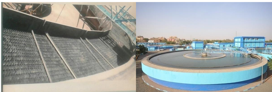
Fig (4.18): Flocculation and Sedimentation basins at Bahri Water Treatment Plant.
