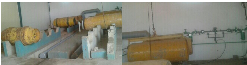
Fig (4.9): Disinfection system at Jabal Awlia Water Treatment Plant.
