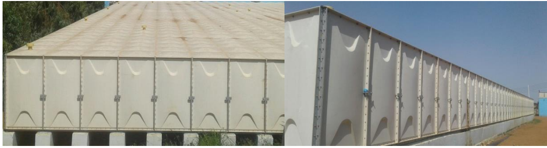
Fig (4.3): Water storage tank at Alshajra Water Treatment Plant
