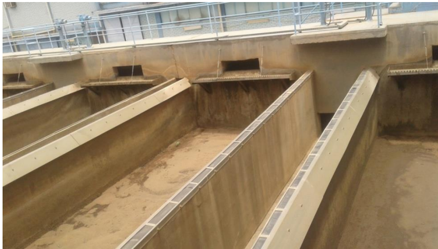
Fig (4.19): Rapid sand filters at Bahri Water Treatment Plant.
