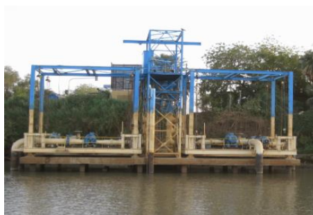
Fig (4.11): Intake at Mogran Water Plant
