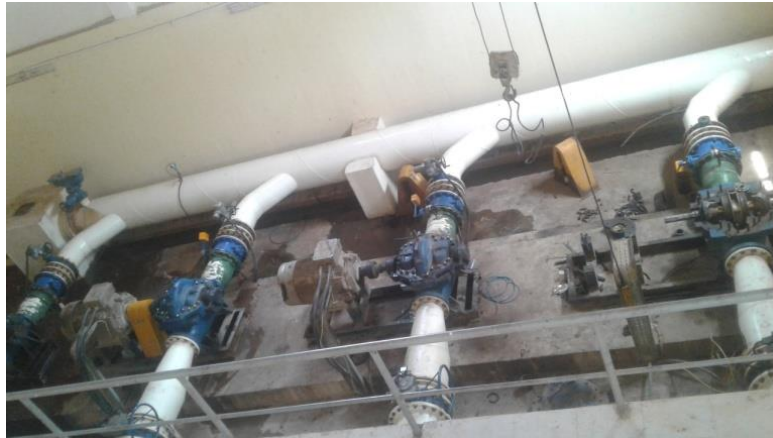
Fig (4.8): low pressure pumps at Jabal Awlia Water Treatment Plant.
