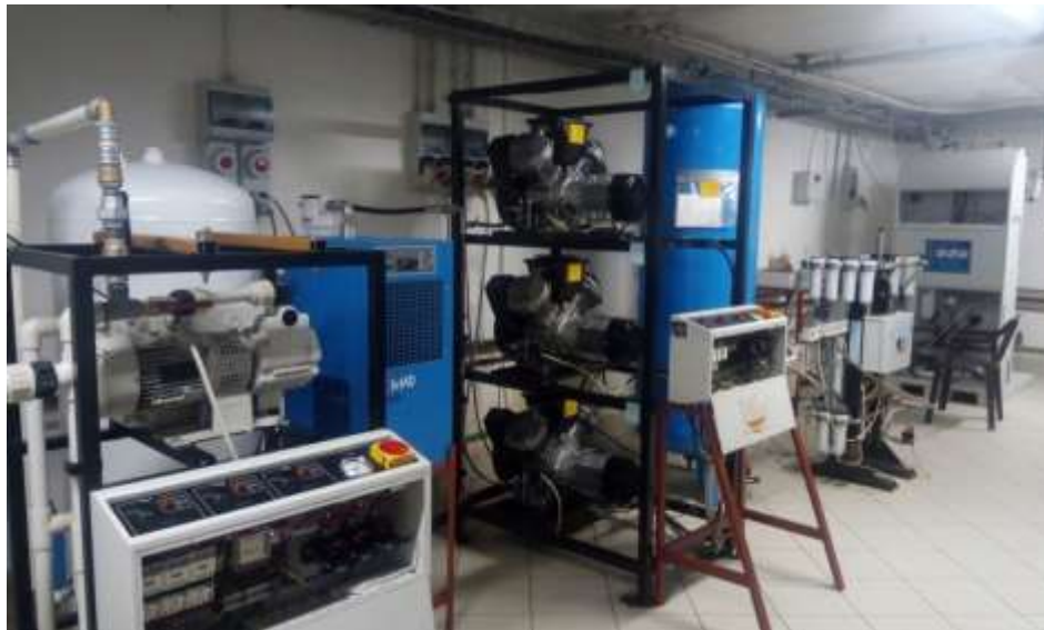
Figure 3-32 part of the Medical Gas System – in basement
