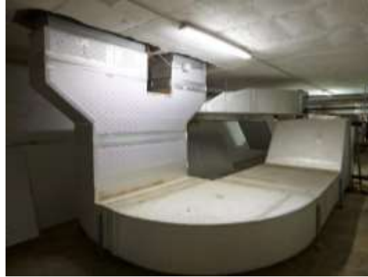
Figure 3-29 Air Handling Unit
