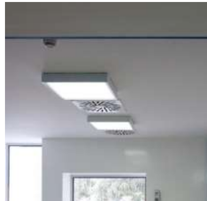
Figure 3-31 Inlet of the Air Supply
