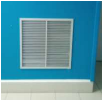
Figure 3-30 Outlet of Air Supply
