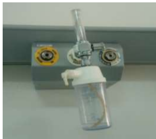
Figure 3-34 Outlet of the system in Wards
