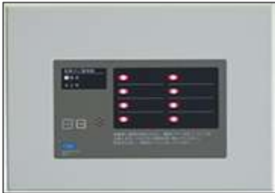
Figure 2-15 Main Alarm Panel
