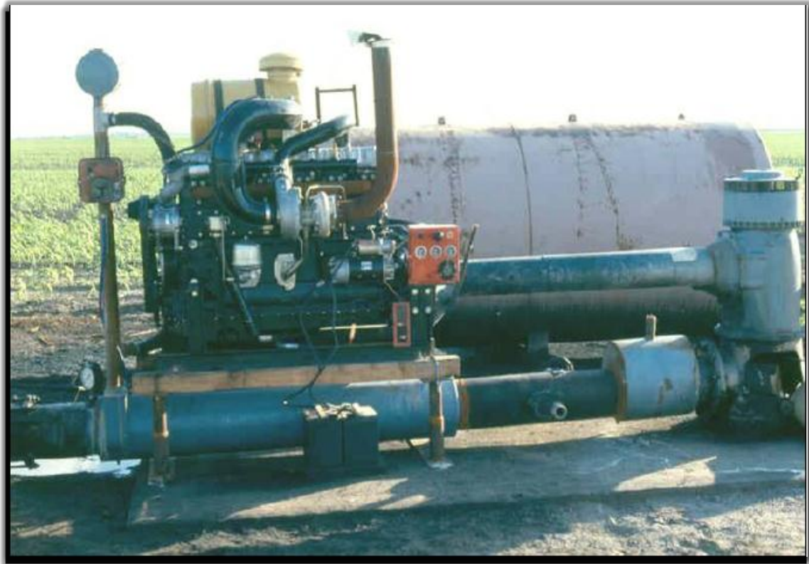
Figure (2.11) Diesel powered turbine pump with right angle drive
