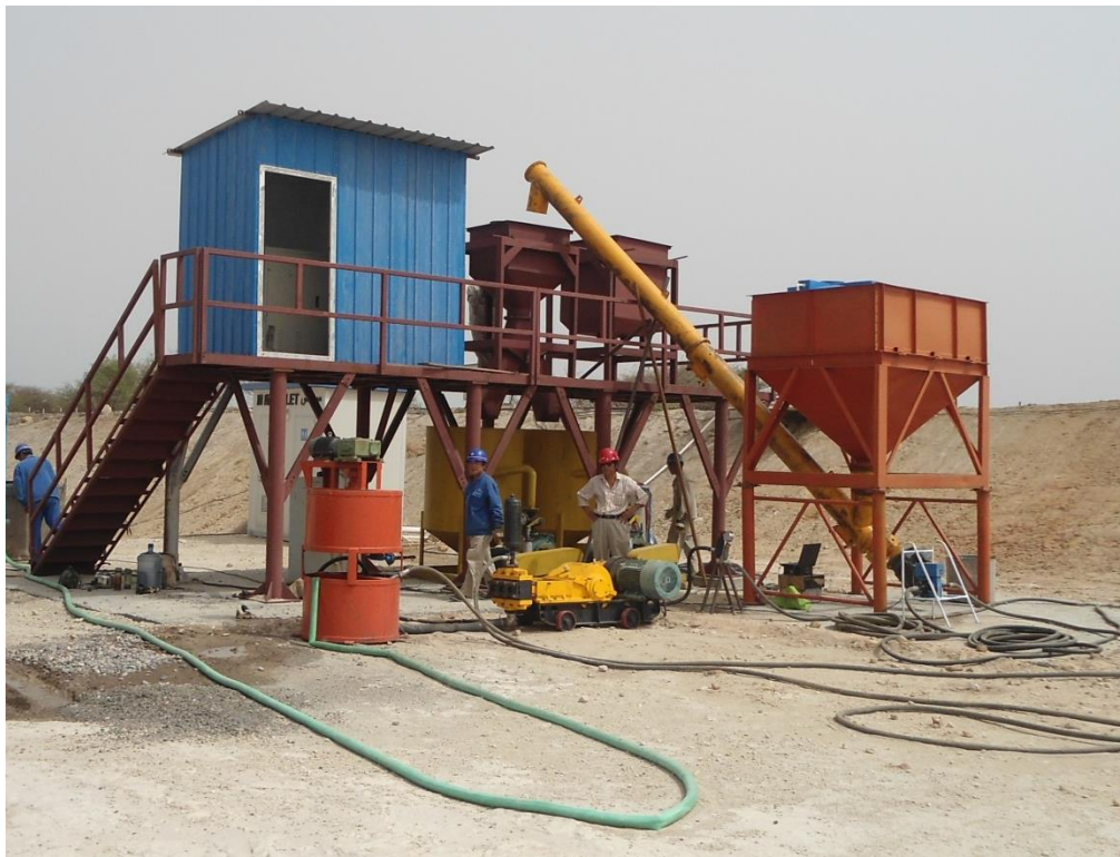
Figure A-13 : JB-1.5 grout mixing plant
