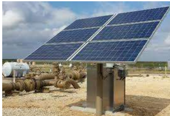
Figure:2.8 Cathodic protection using PV
