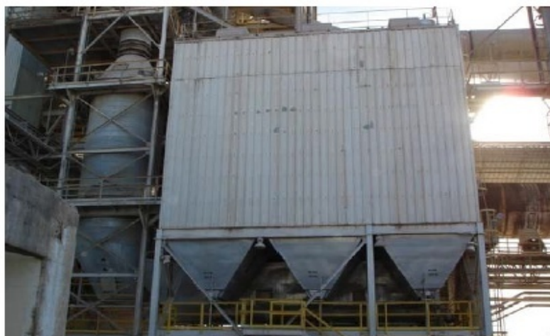
Figure 2.6 Dust control device (Courtesy of Capitol Cement) [3]
