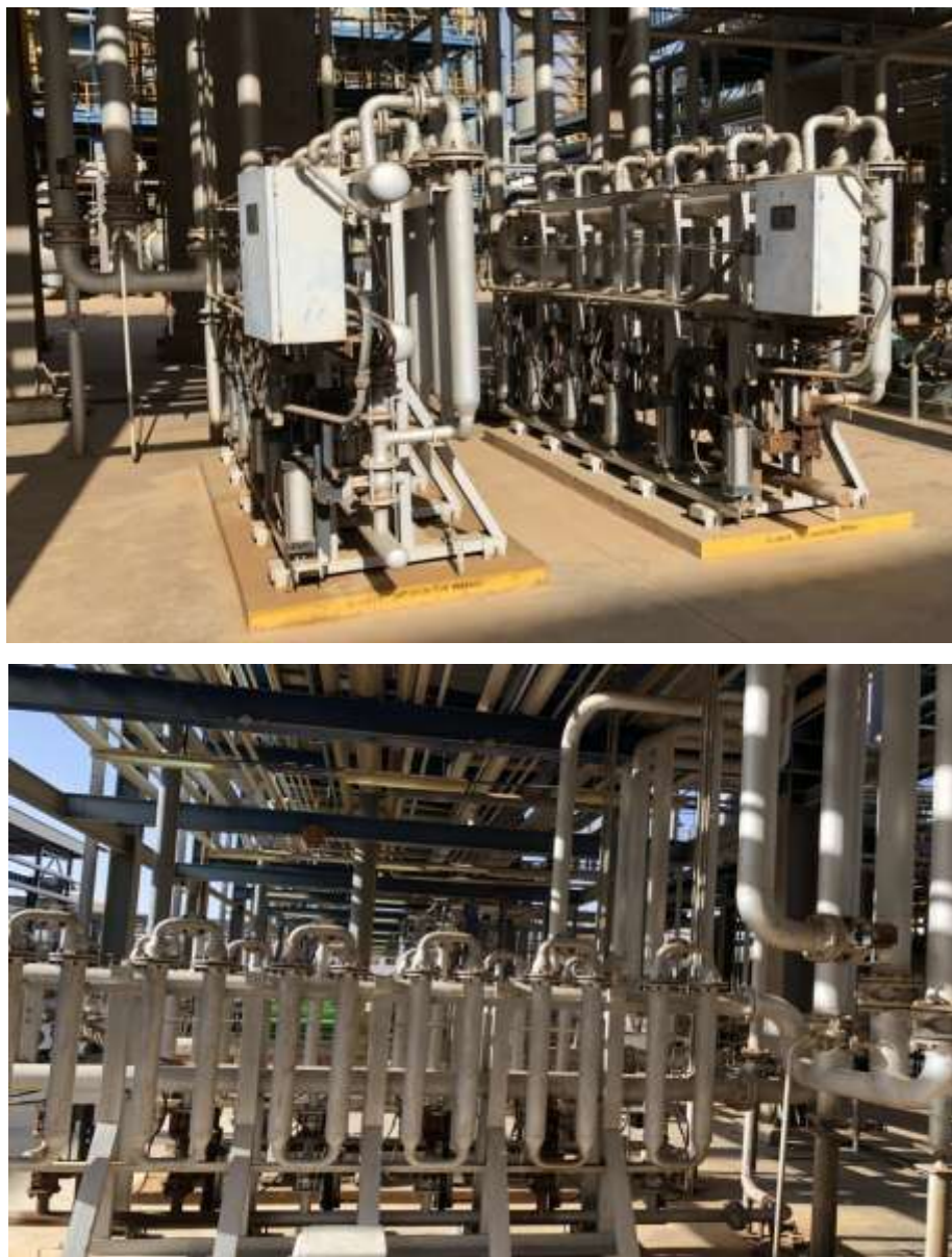
Figure 2-1: DHT Unit Backwash Filters
