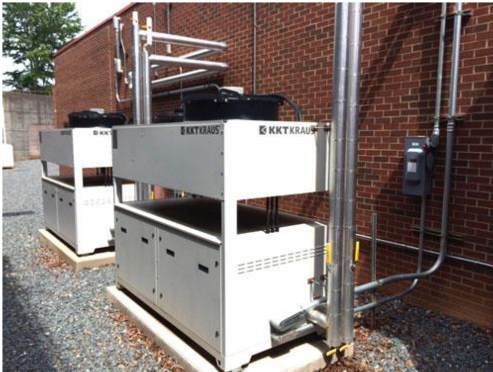
Figure 2.13 Chiller (outside components)
