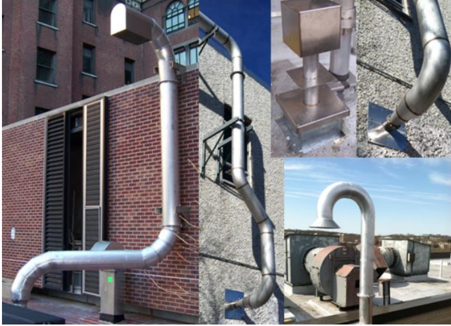
Figure 2.18 MRI quench pipe
