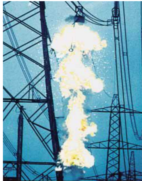
Figure 2.2: Possible consequence of inadequate protection
