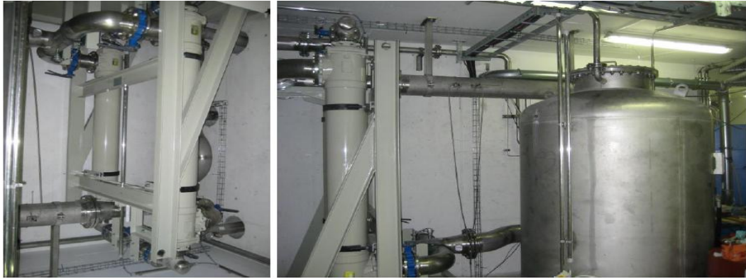
Figure 3-12 External oil tank and coolers
