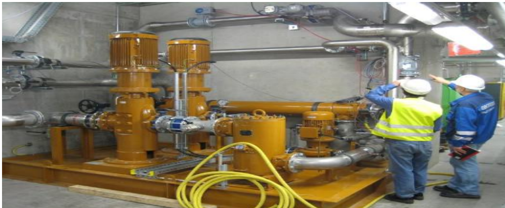
Figure 3-11 External water cooler
