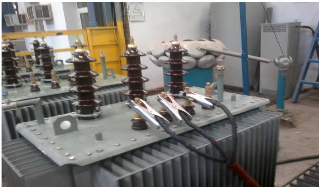
Figure 3.4: Transformer under open circuit test
