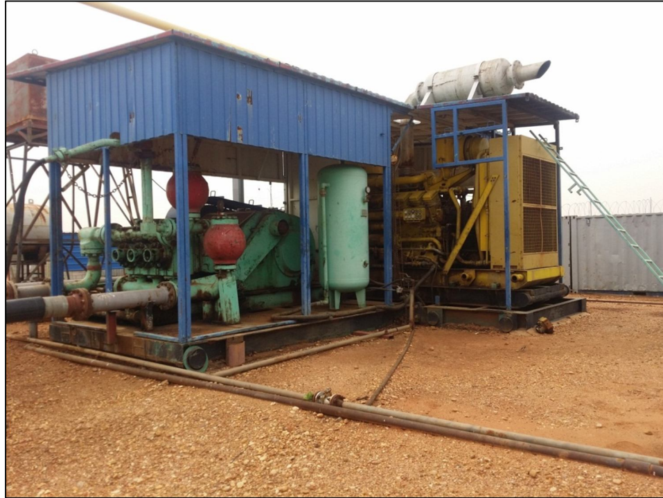
Figure 2-2: mud pump compartment other view.(Baoji, 2005)
