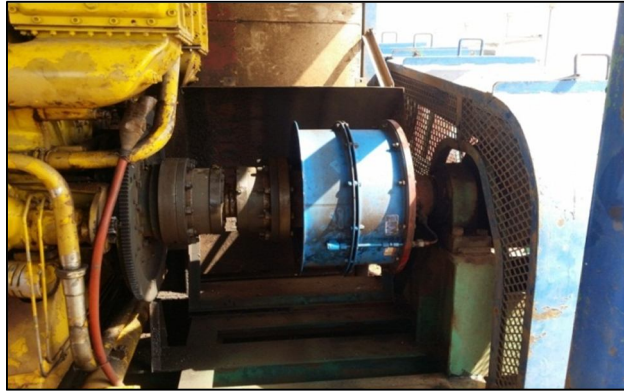
Figure 2-8: Air clutch installed in the unit.(Baoji, 2005)
