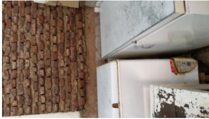
Figure 9 : Absence of ceramic or wall insulation
