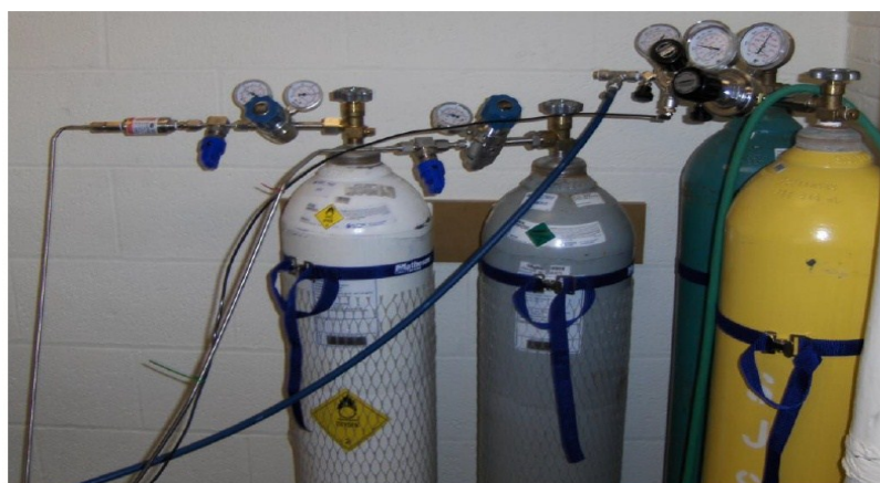
Figure 6: Gas tanks (left to right: O 2 , Ar, “low” purity Ar, and Air) and associated hardware
