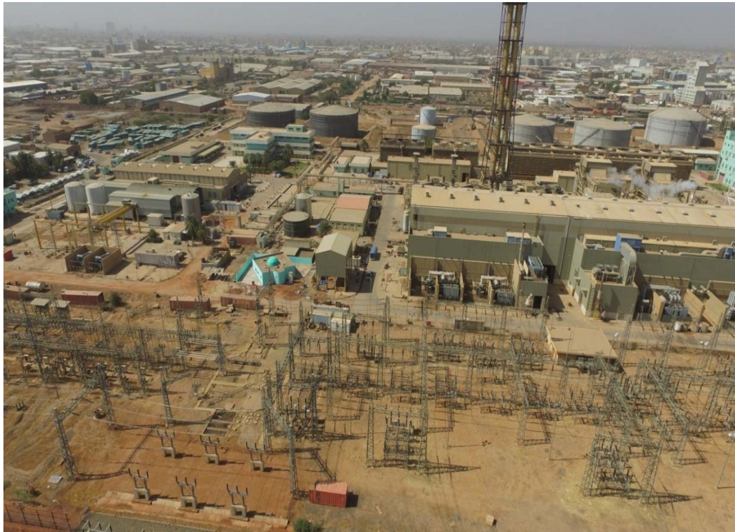
Figure 2.1: Khartoum North Power Plant Station.
