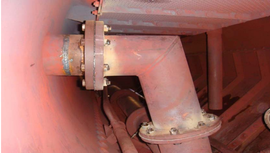
Figure 2.12: Internal side of boiler drum.
