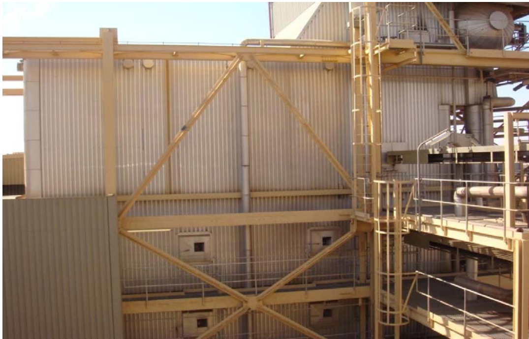
Figure 2.16: over all outside of boiler.
