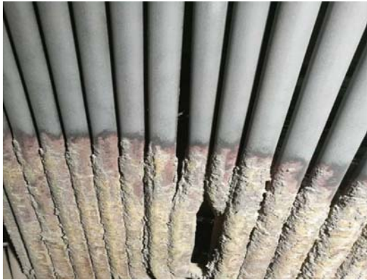
Figure 2.25: Water wall Fireside Corrosion.
