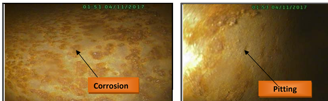
Figure 4.4 -A: Corrosion inside tube Figure 4.4 -B: pitting inside tube
