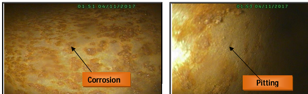
Figure 4.4 -A: Corrosion inside tube Figure 4.4 -B: pitting inside tube
