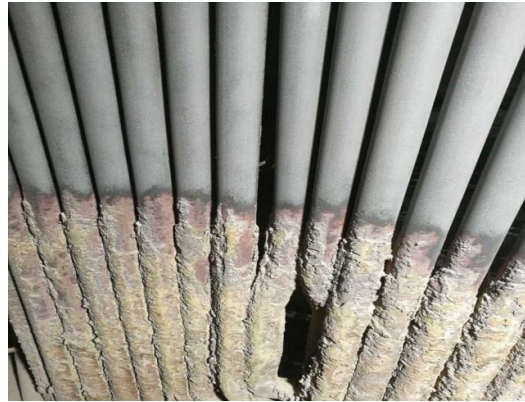
Figure 2.25: Water wall Fireside Corrosion.
