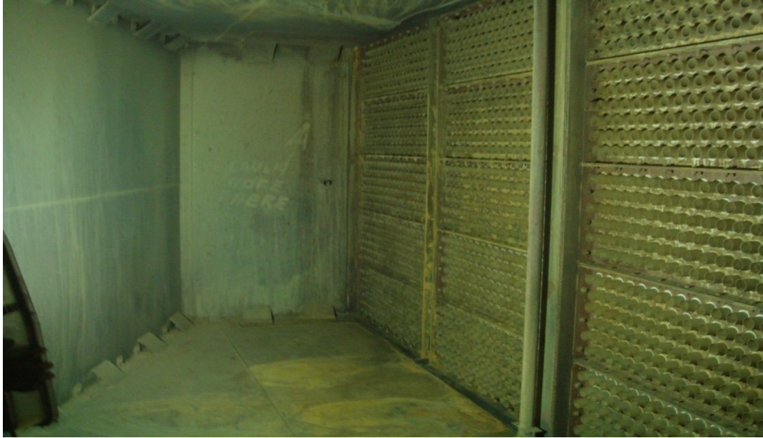
Figure 2.13: Internal side of Air heater.
