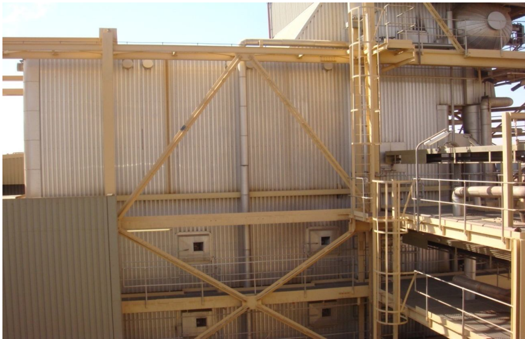
Figure 2.16: over all outside of boiler.
