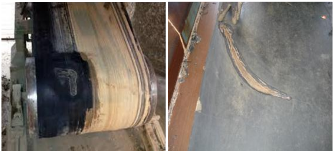
Figure (2.2) Belt Damage
