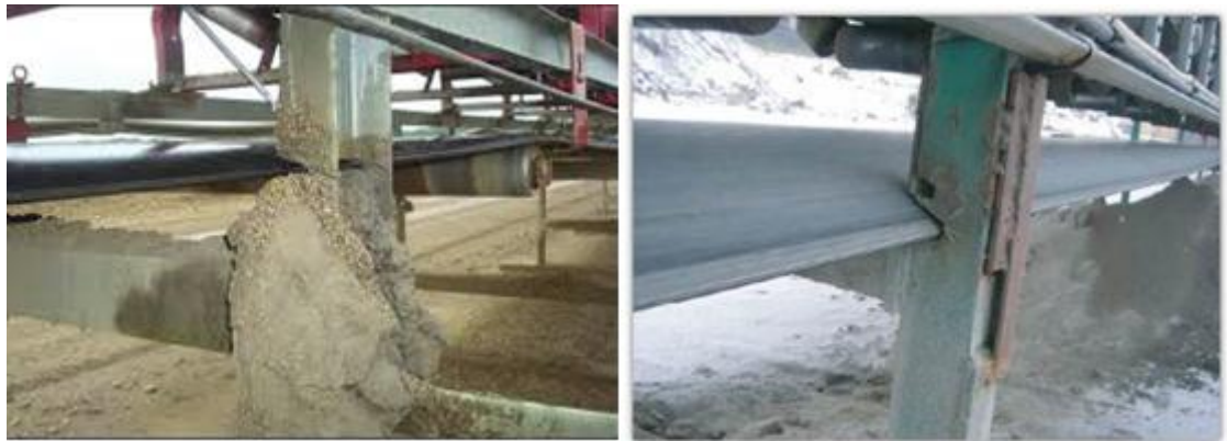
Figure (2.1) Structure Damage
