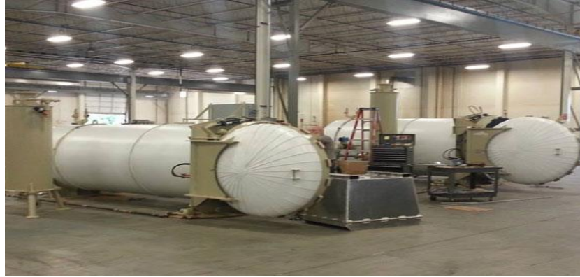
Figure 2.6 show incinerators with two chambers [24].
