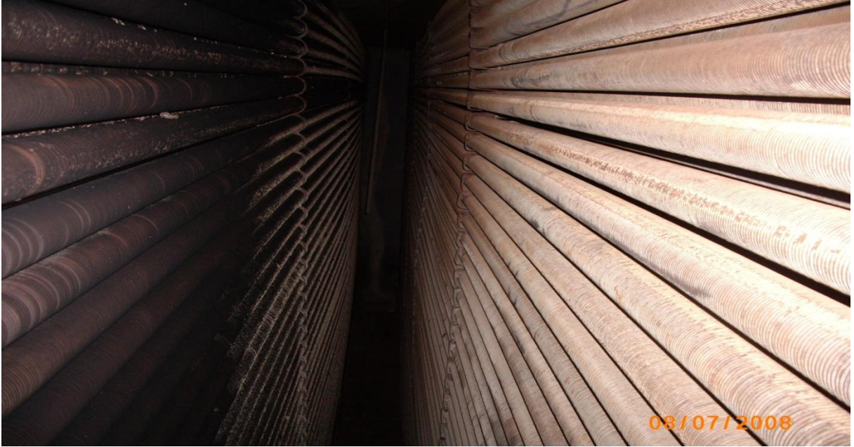
Heat Recovery Steam Generation Pipes
