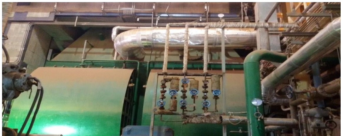
Figure3.5: surface condenser in unit six
